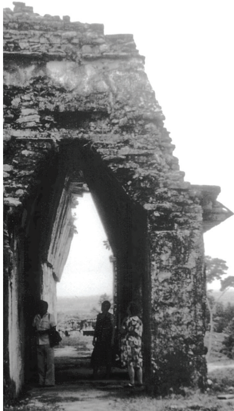
Figure 3: An Arcade at Palenque: space in a thick wall. (From a colour photo by Ranulph Glanville)
